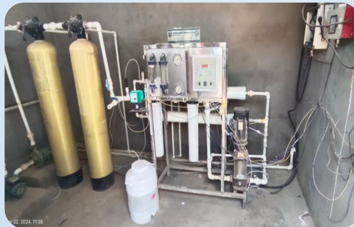
Installed RO based-Drinking Water Cooler in Durga Public School, Dachehalli, Andhra Pradesh.
