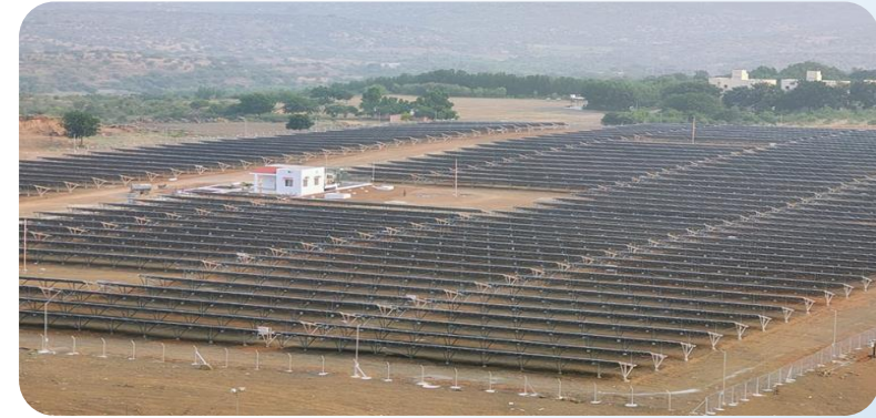
6 MW Solar Power Plant, Gudipadu, Andhra Pradesh
