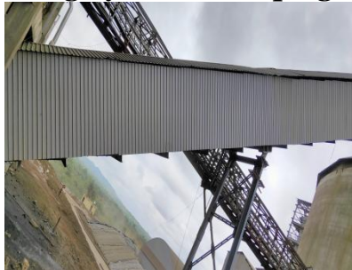
Covered belt conveyor
