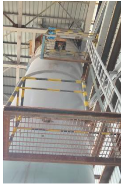
Opacity Meter(Cement Mill Stack)
