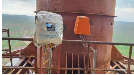
Opacity Meter(RM+Kiln Bag house Stack)
