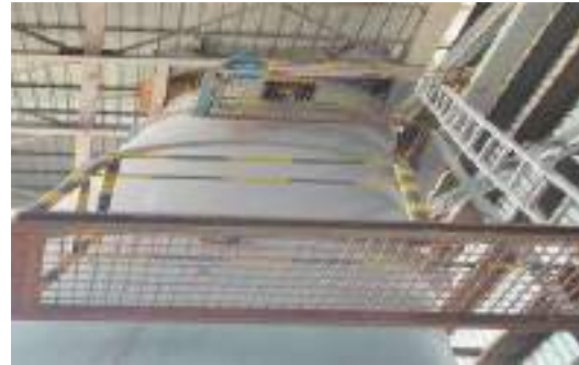
Opacity Meter (Cement Mill Stack)
