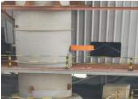
Opacity Meter(Coal Mill Stack)
