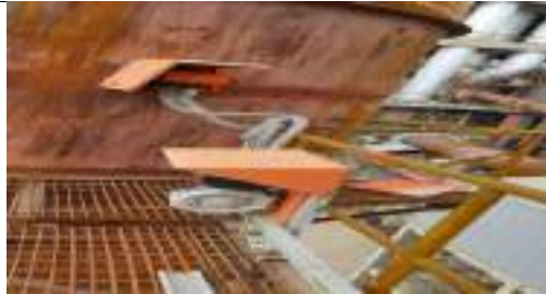
Opacity Meter(Cooler ESP Stack)
