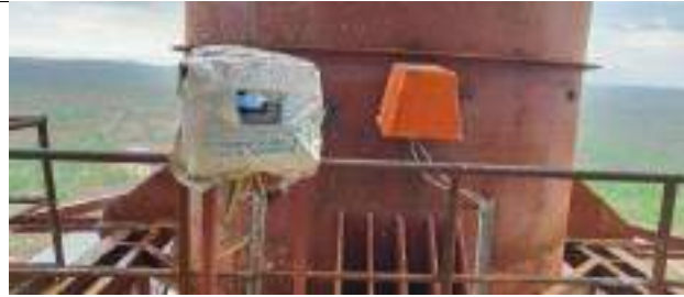
Opacity Meter (RM+Kiln Bag house Stack)
