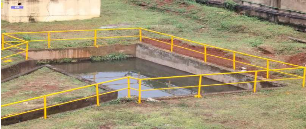
Rainwater Harvesting pit
