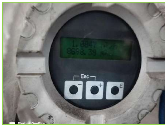
Process Water Meter
