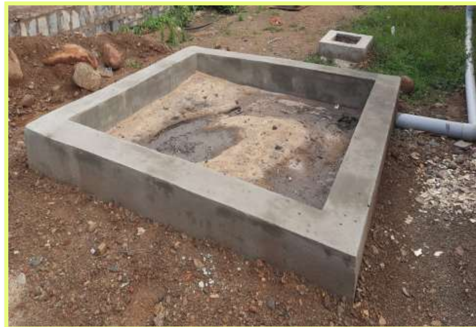
Rain water harvesting pit near Plant area
