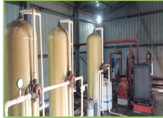
Water Purification Plant
